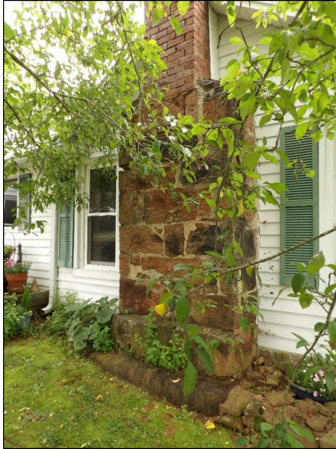
Photo 5: Composite Masonry Chimney on the South Elevation of the Original Log Section, Looking Northwest.
