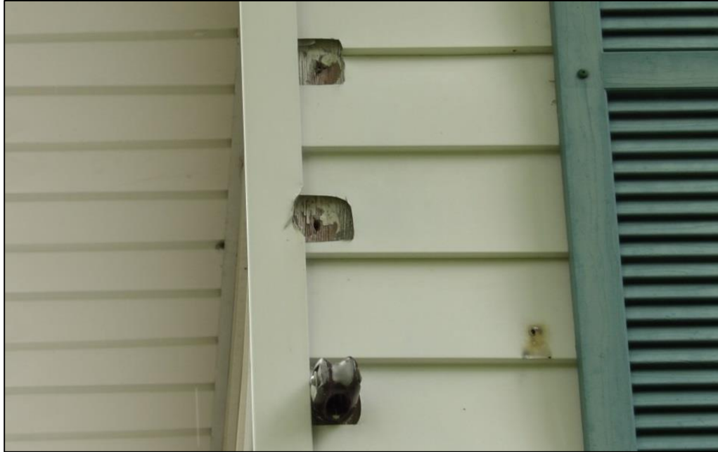
Photo 10: Exposed Wood Siding Visible Through Holes Cut Into the Vinyl Siding on the Second Story of the North Elevation, Looking South.
