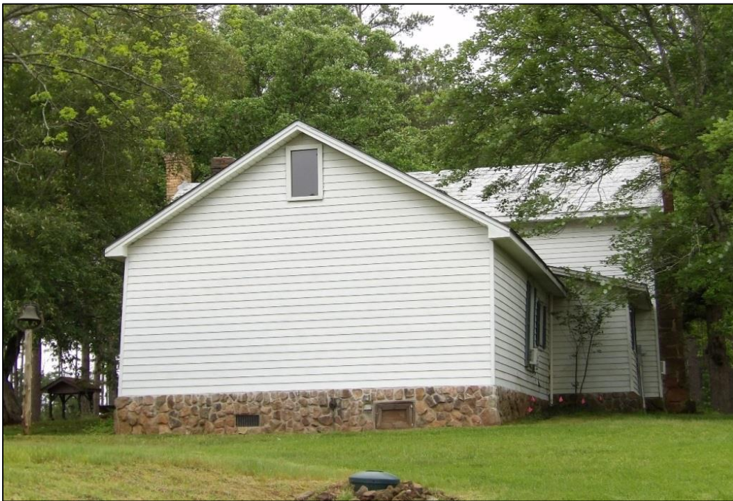
Photo 4: East Elevation of Log Section Showing Vinyl Siding and Brownstone Veneer Obscuring Foundation.
