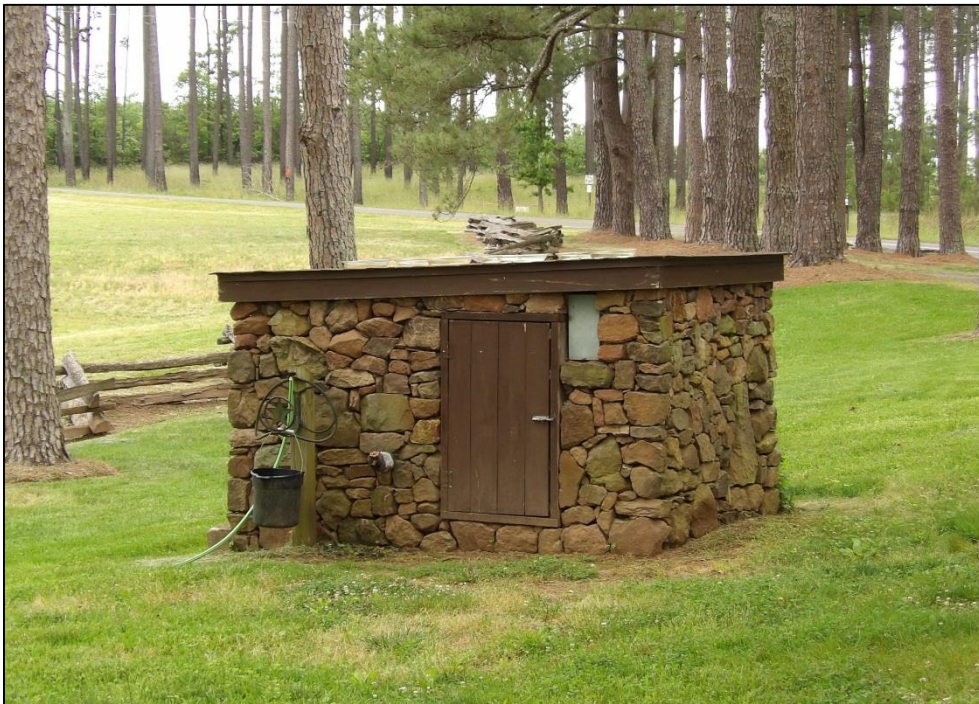
Photo 21: Large Well Head, Looking Southwest.
