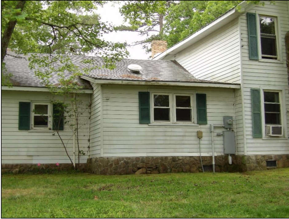
Photo 17: Shed-Roof Projection on the North Elevation of the One-Story Addition, Looking South.
